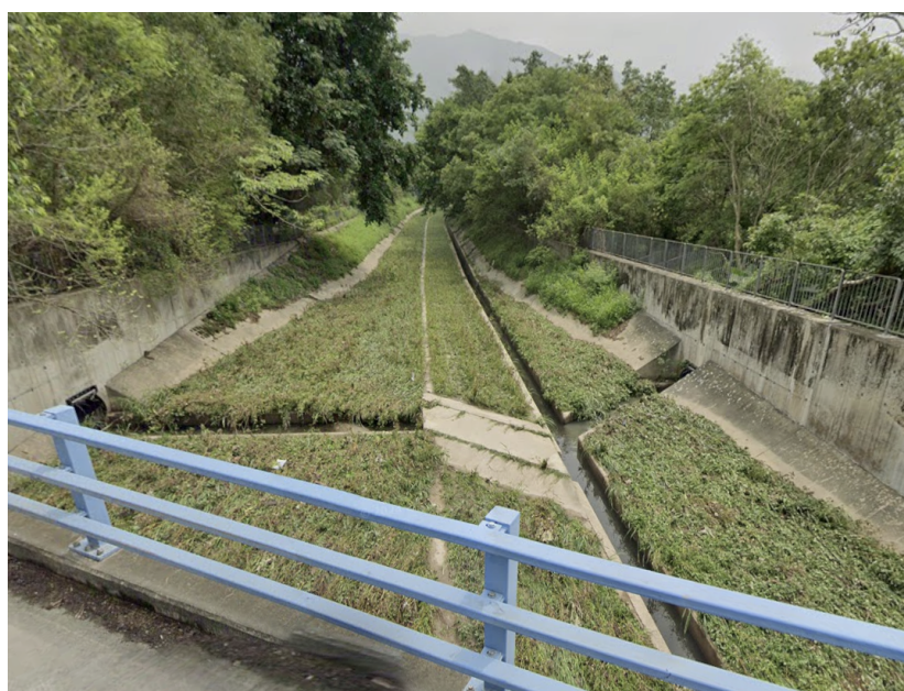
Final Discharge Point
